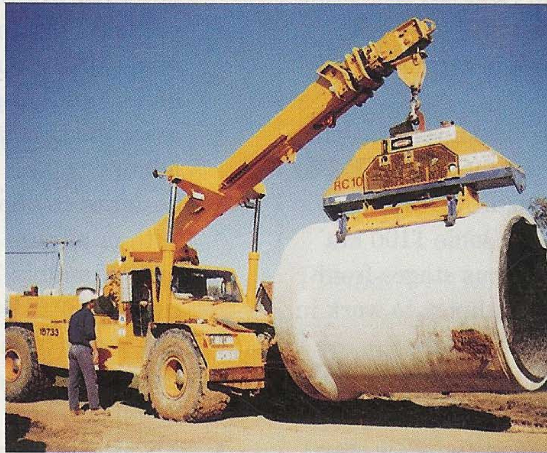
The self contained RC10 lifter handled 1950 mm dia. concrete pipes for the Water Authority of WA.
